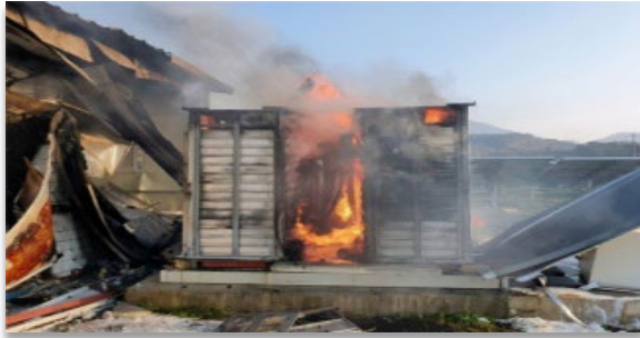
Only the fire extinguishing system extinguishes the fire, and there is no pre-accident risk warning in South Korea's energy storage accident.
